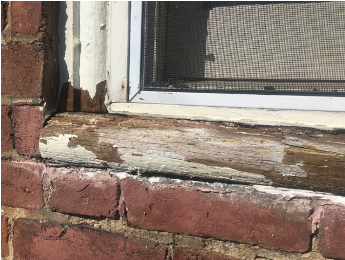
This section is in the best shape. You can see bits of the wood filler left in some of the horizontal
