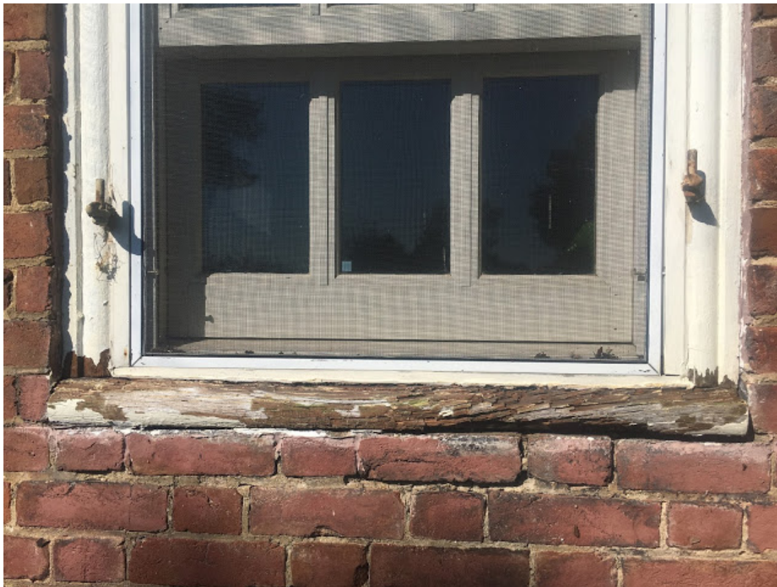
This is what the sill looked like after removing the peeling paint. The shape is meant to be a bullnose, but so much wood is deteriorated, there isn't much original shape left.
