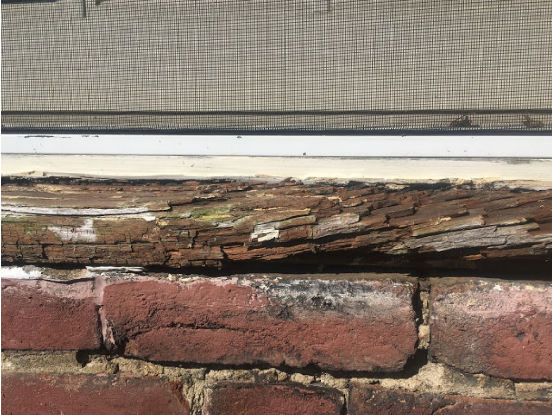
A close-up of the most damaged portion.
